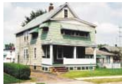
Enclosure of second floor porch has disturbed the structural and visual balance of the home. The second story dominates and looks out of proportion to the first story.
